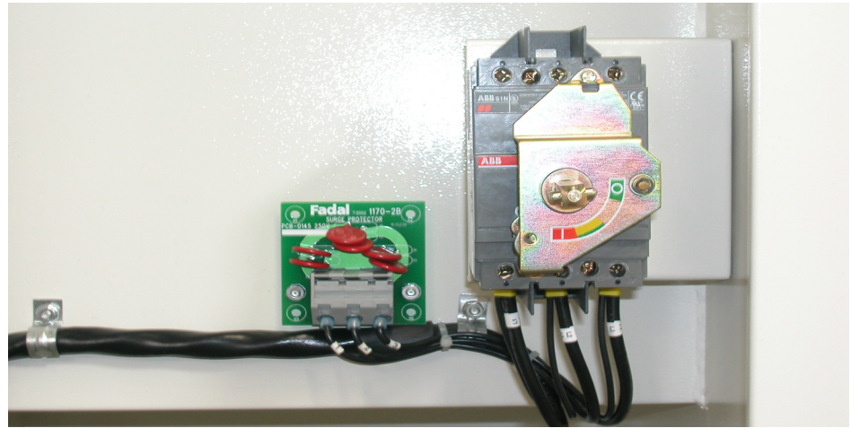
Figure 3-2: MOV Surge Suppressor Board
