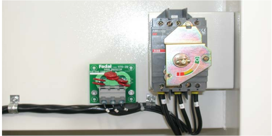
Figure 3-2: MOV Surge Suppressor Board
