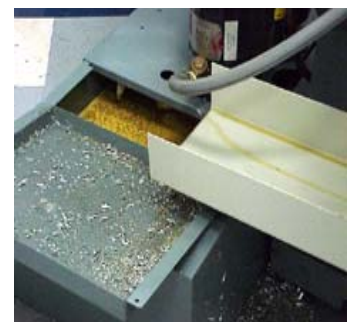
Figure 1-3 Coolant tank fill level.
