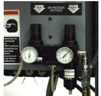
Figure 1-2 Air pressure gauges.
