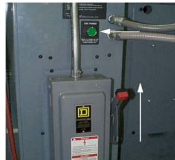
Figure 1-5 Main power box and green power button.
